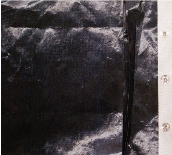
ABOVE: Belt is torn and folded. Replace belt.
