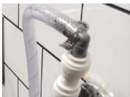
Figure 8. Soft Water Outlet from Water Softener to Steamers with Shut Off Valve.
